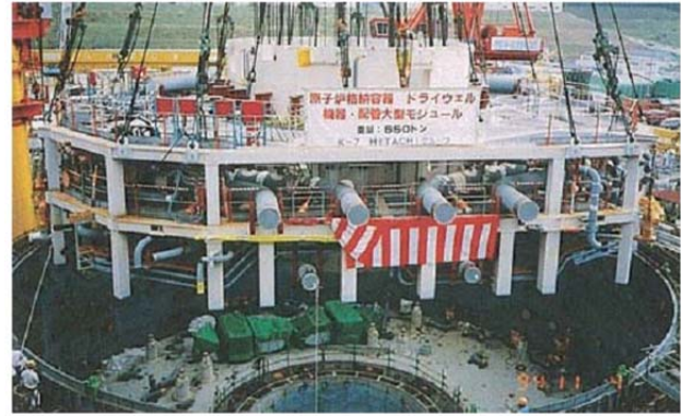
Installing The Upper Drywell Super Large Scale Module At Kashiwazaki Kariwa-7 In Japan:
